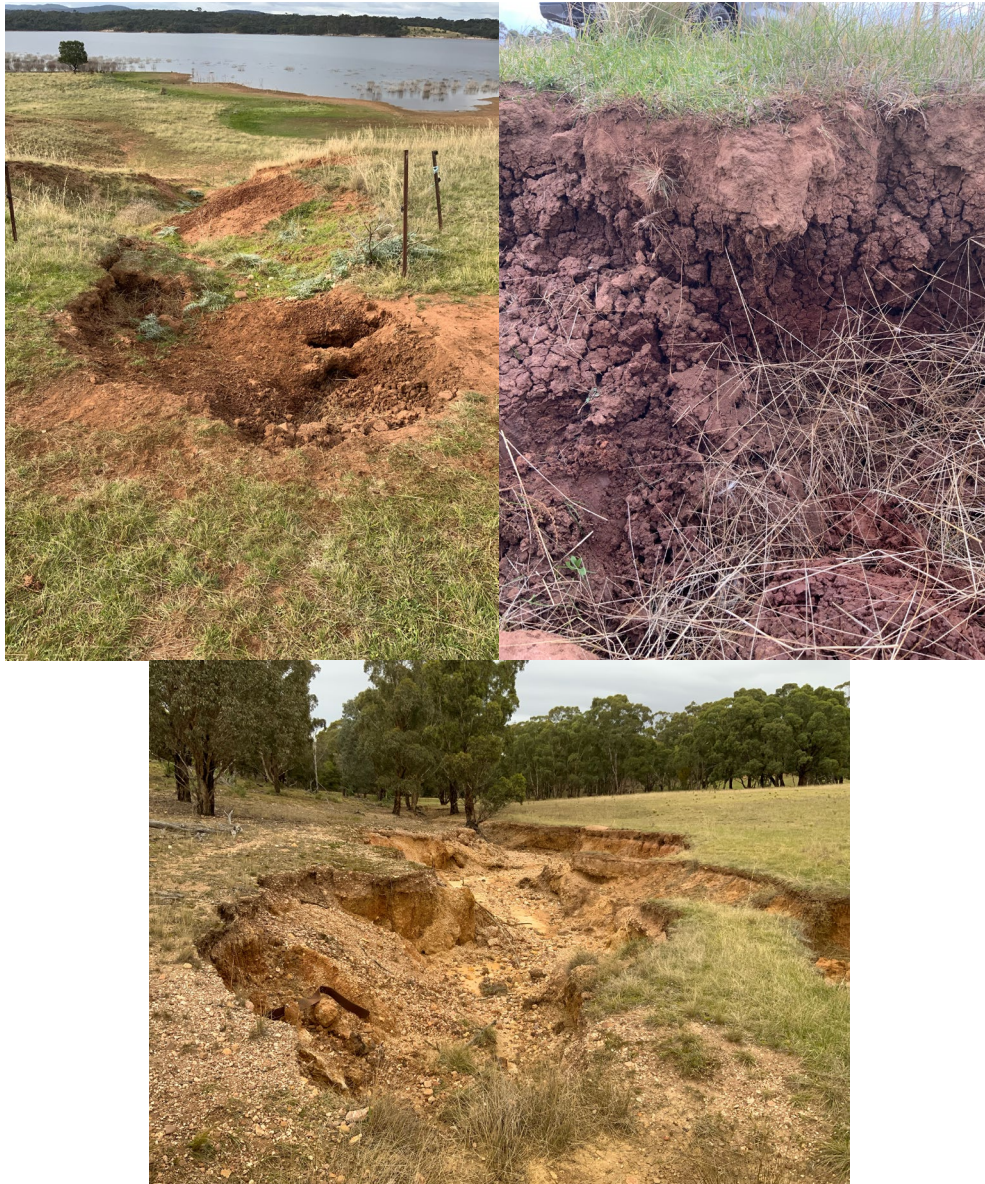
Figure 11. Merrimu Reservoir erosion areas.
