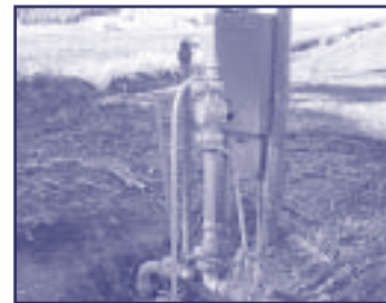
Newly-installed groundwater meter
