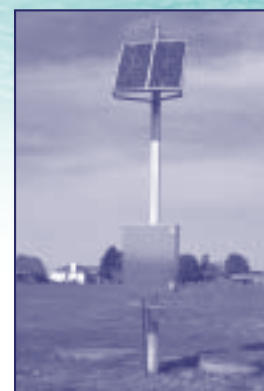
Technology to measure permanent pressure levels in the Boisdale pipeline
