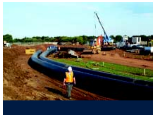
■ Above: Replacing the Bacchus Marsh flume Below: Western Irrigation Business HDPE pipeline project
