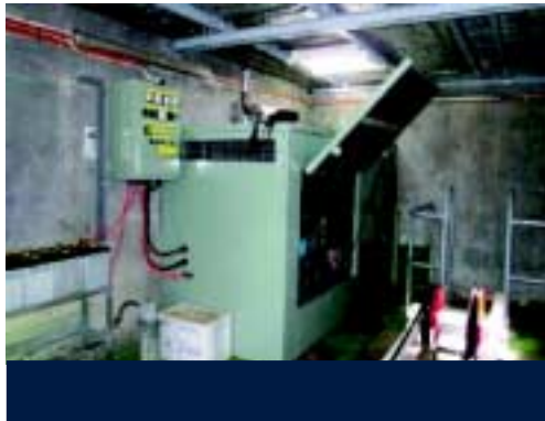
■ Our new Lerderberg diesel generator
